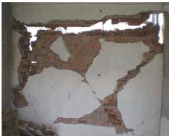
Kutahya Earthquake, Turkey May 29, 2011
