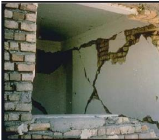
Manjil Earthquake – Northern Iran, June 21, 1990
