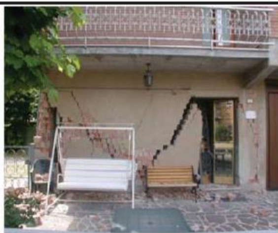
Emilia Earthquake – Northern Italy, May 20, 2012
